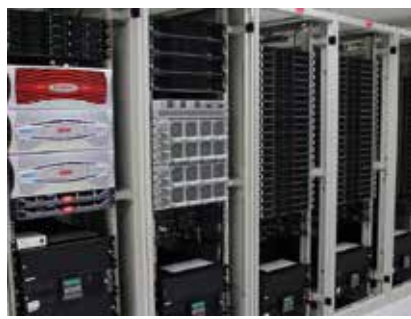
Computation server (Internet Architecture and Systems Lab)
