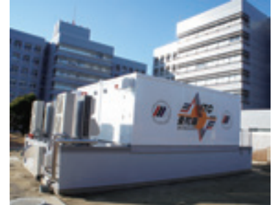
Container server room (Information Initiative Center)
